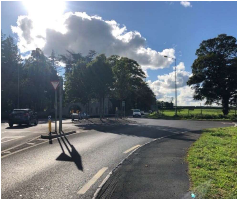
Location 10 - N21 L1420 L1424 Roundabout Direction Continue Straight On N21 Visual inspection indicates Road widening required on offside of entering and exit of the roundabout Swept path analysis recommended to confirm this
